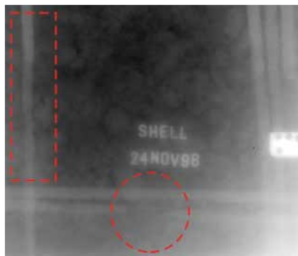
Fig. 4: Severely corroded reinforcing bars
